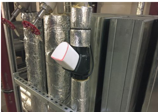
The retrofitted Hycleen Automation System guarantees reliable drinking water management at consistent temperatures above 55°C and a hydraulically balanced installation.
