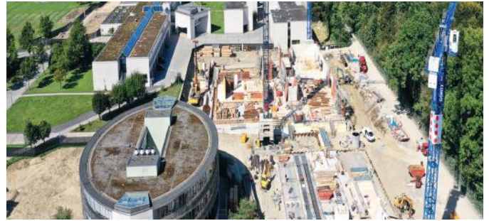
Expansion of the second largest weapons site in Switzerland. Image: armasuisse Immobilien. Image title page: VIZE architectural rendering. Architecture: Baumschlager Eberle Architects
