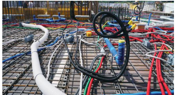
The iFIT pipes (black) are fitted for the drinking water supply to the apartments.
