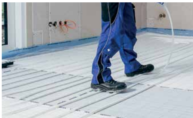
The intermediate spaces are filled with Uponor KLETT panels and the underfloor heating pipe is laid quickly and easily over the entire area of the room.
