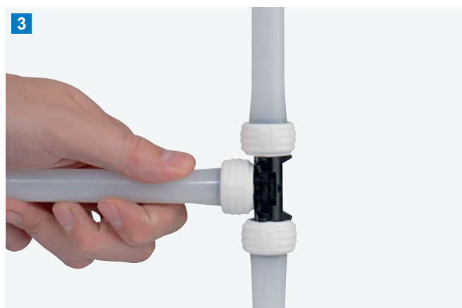
Remove the expanded assembly from the tool and place on to the fitting, holding the whole assembly for a few seconds until the pipe starts to shrink down on to the fitting.
